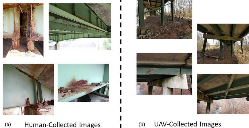
Fig. 3. (a) Human-collected (Bianchi and Hebdon 2021b) versus (b) UAV-collected images of corrosion on a bridge in Douglasville, Georgia.
